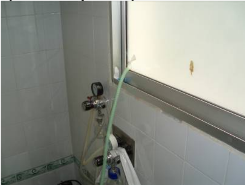
Figure 5: extended t-piece scavenged out of the window
